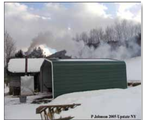
Outdoor wood boiler in Upstate New York
