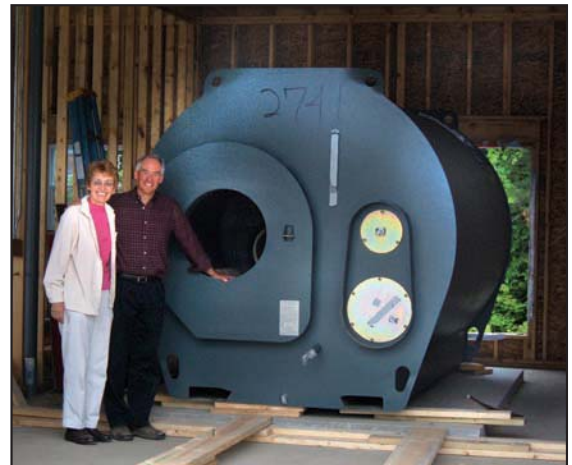
Photo courtesy of Ave Maria Community Care Homes Steven Doe and Claire Doe pose with the new wood-fired Garn boiler at Our Lady of the Meadows in Richford. It is just one of the energy-saving facets of the nursing facilities expansion project.
